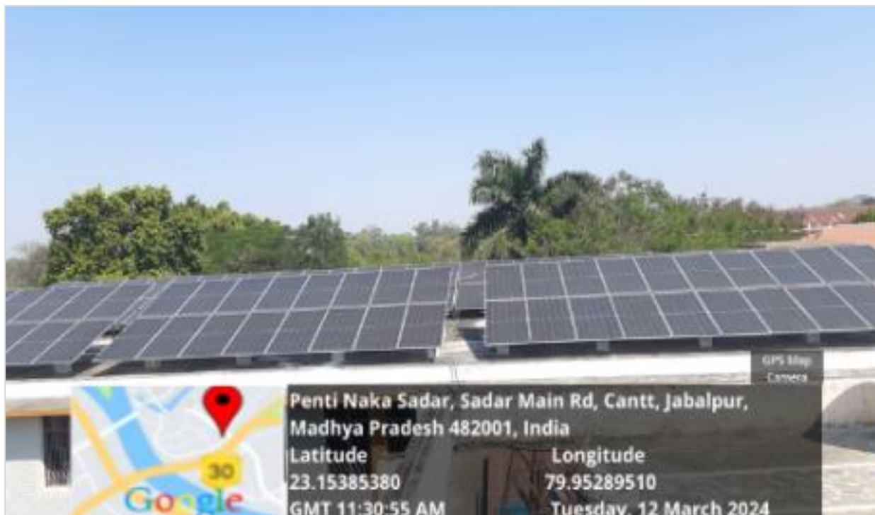
Plate 1: Rooftop solar panels in the premises
